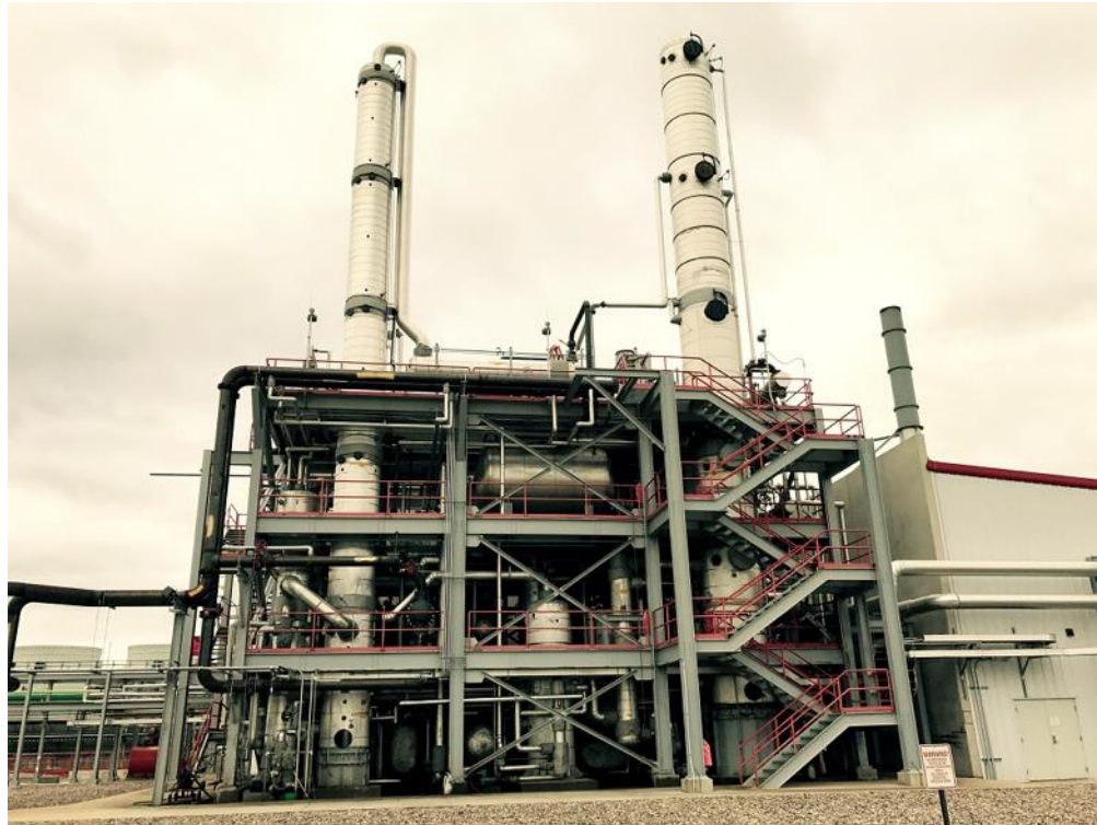
Patriot Renewable Energy, biodiesel plant (now owned by CHS, Inc.), Annawan, IL
